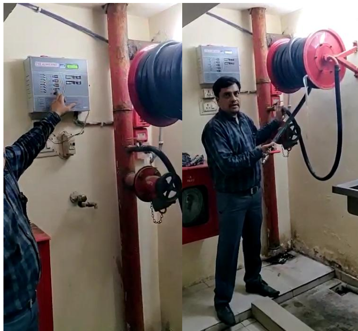
Faculty explaining about A-block fire safety system
